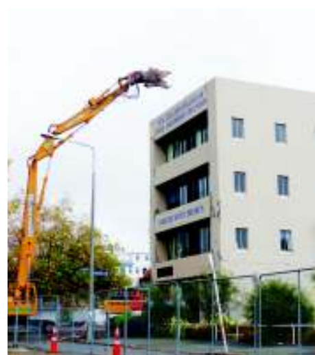
Due for Demolition, Early Childhood Education Building, 50 Victoria Street, Christchurch
